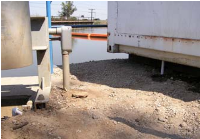
Out the container via a buried pipe...
