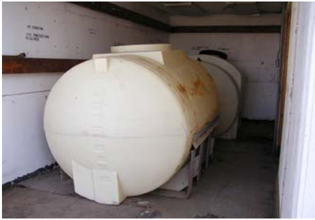
2 x 500 gallon tanks inside secure 20 ft container
