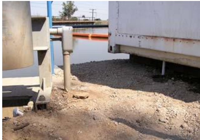
Out the container via a buried pipe...
