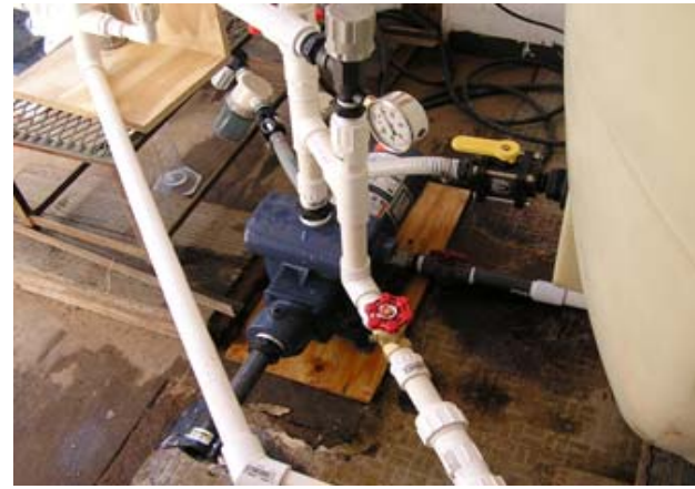
Pump canal water into both tanks
