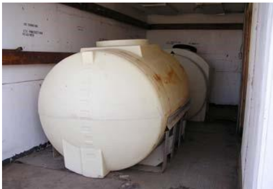
2 x 500 gallon tanks inside secure 20 ft container
