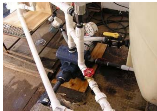
Pump canal water into both tanks
