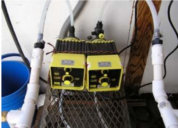
Independently meter both solutions from tanks...
